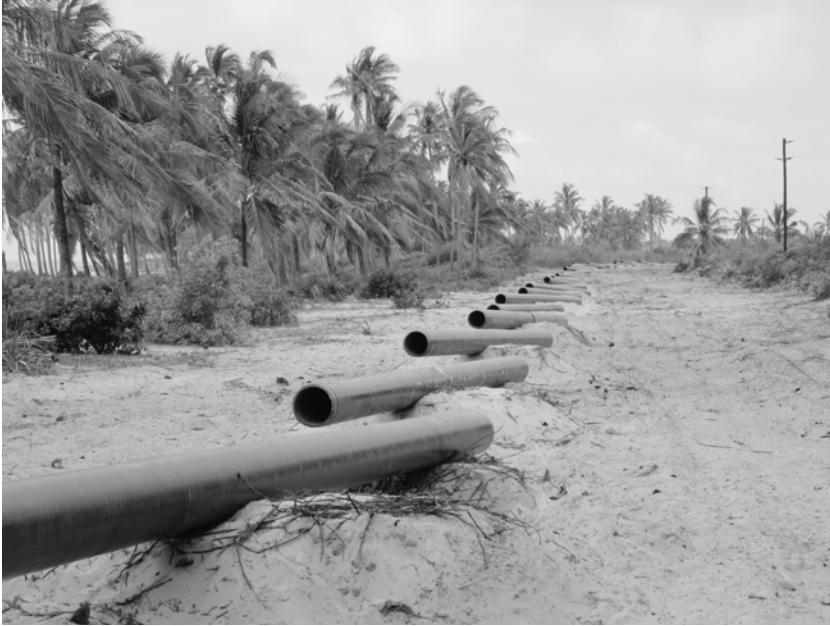
FIGURE 8 Gas pipeline along the Msimbati oceanfront in August 2014
